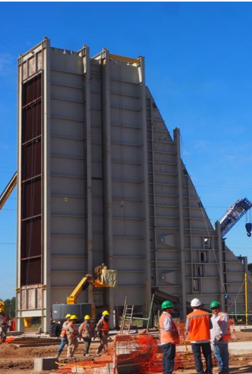
Arroyo Seco Power Plant
