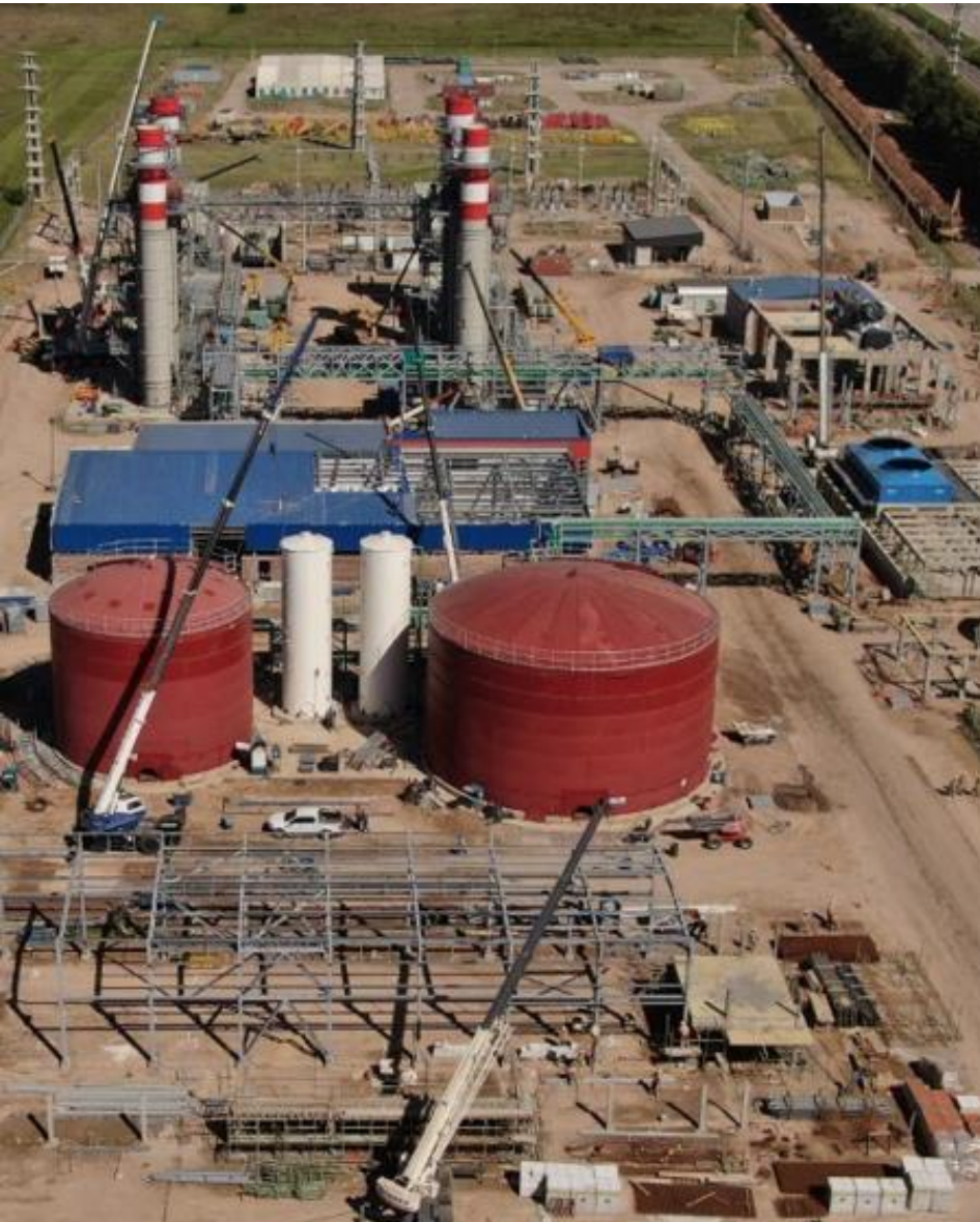
Arroyo Seco Power Plant
